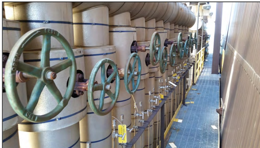
Missing tags on valves
