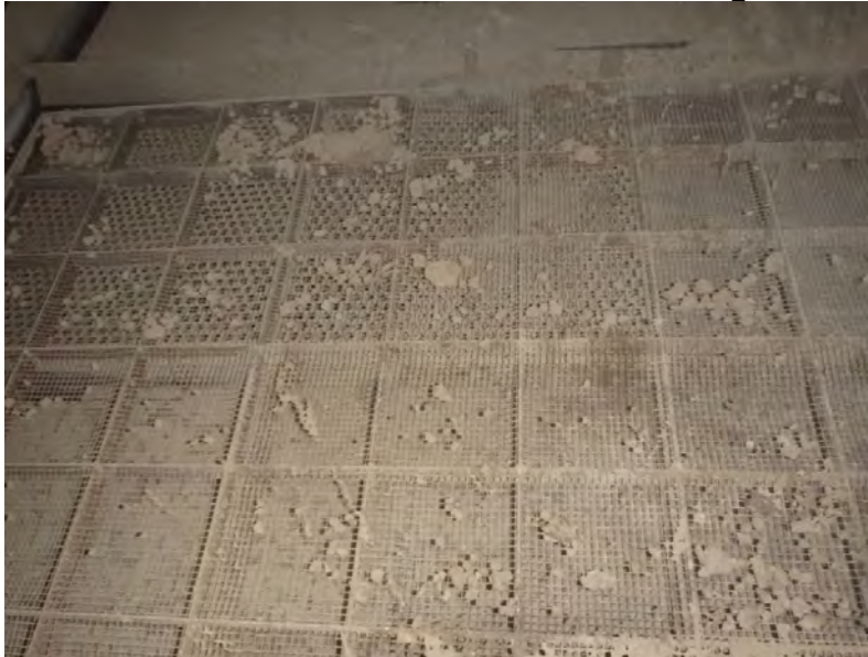
Severe Erosion in L1 after 56,000 hrs
