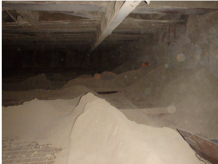
Ash Piles in L3
