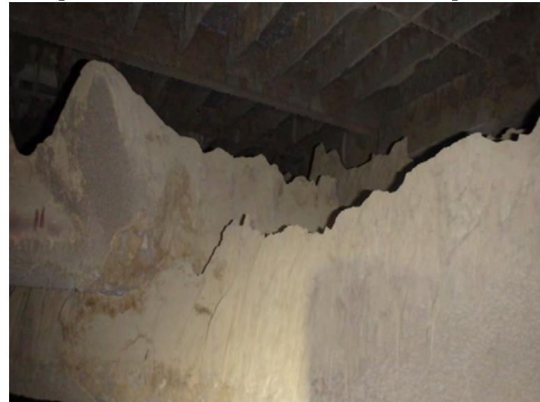
Large Accumulations on Trusses/Beams
