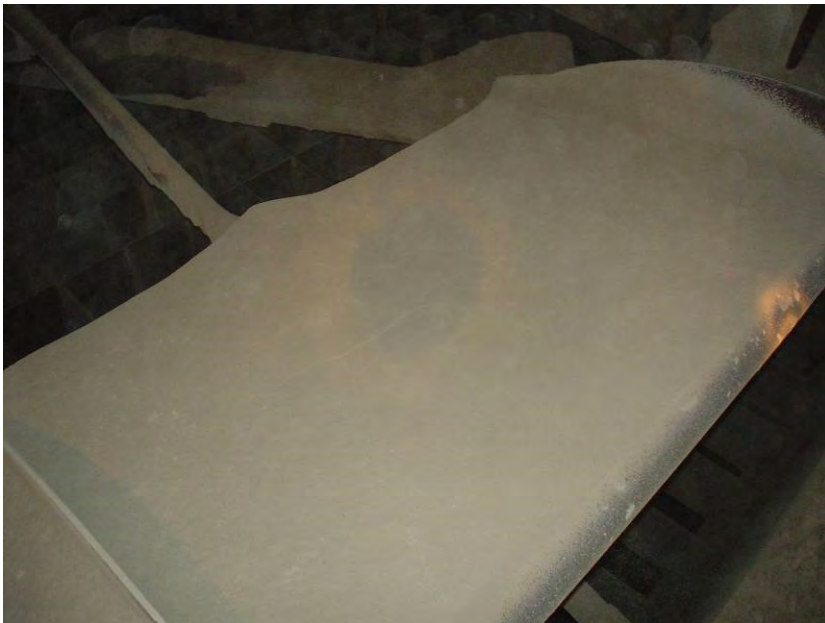
Ash Buildup on Vanes
