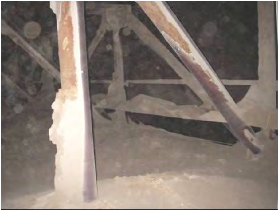
Ash buildup in crossover duct
