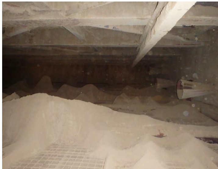
Ash Piles in L4
