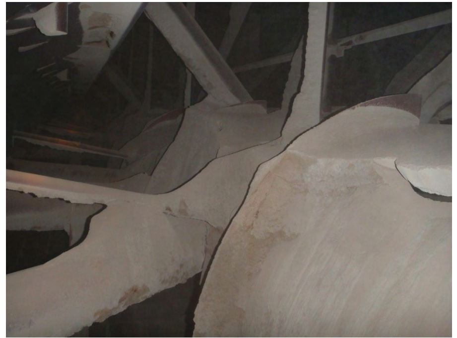
Ash Buildup “Dirty” Condition
